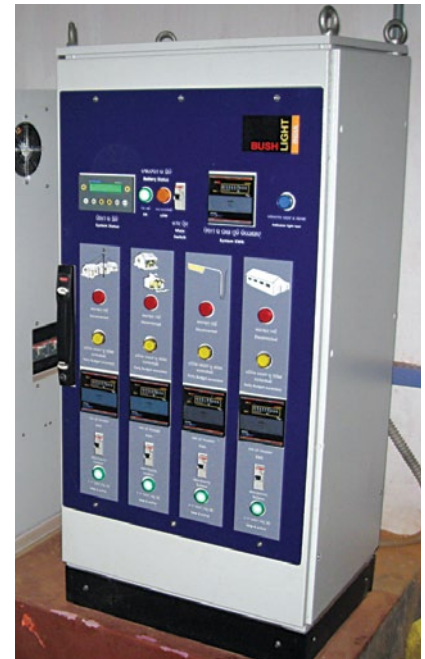
System Control Board
