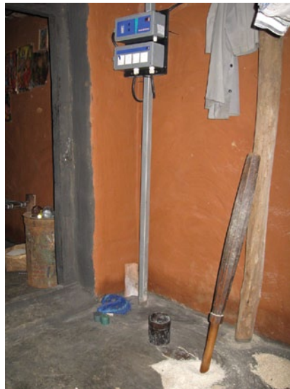
Urja Bandhu installed on stand-alone mounting pole in a house in the village of Maligaon, Orissa.
